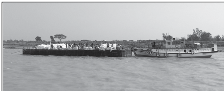
Phase-II work for nourishment and re-building of spurs at Nischintapur is in progress
