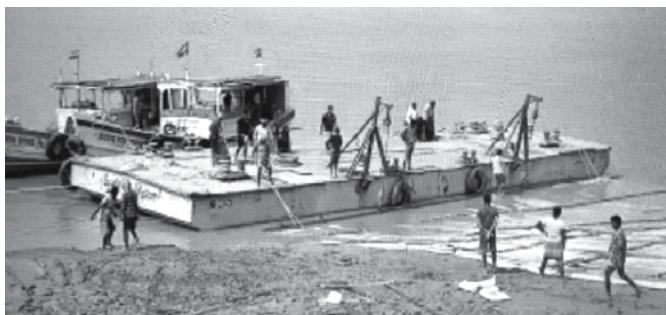
Phase-I work for nourishment and re-building of spurs at Nischintapur is in progress
