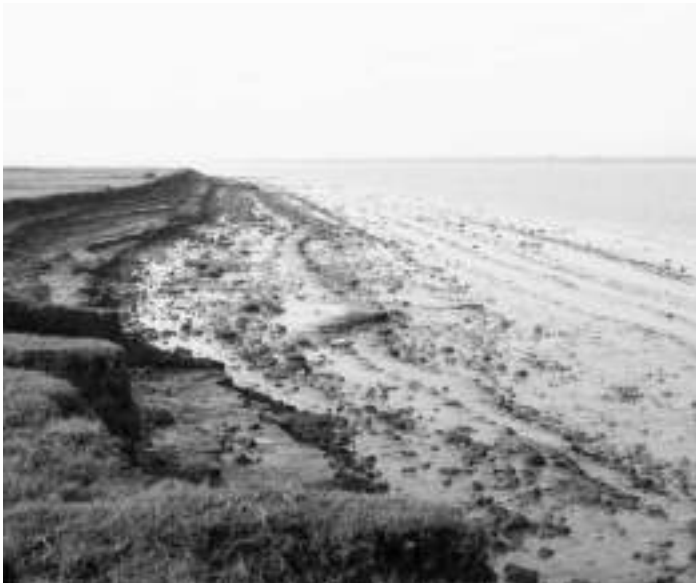
Erosion at Shalukkhali
