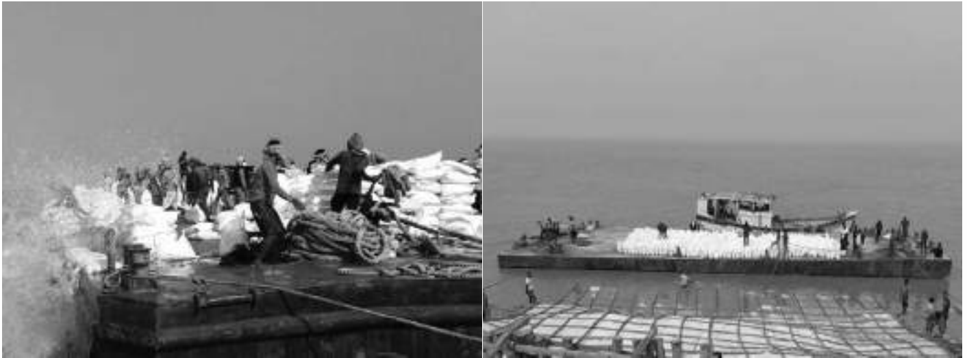
Work of nourishment and re-building of spurs at Nischintapur is in progress
