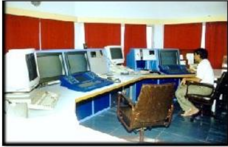
Figure I: VTMS Control Room at Haldia
