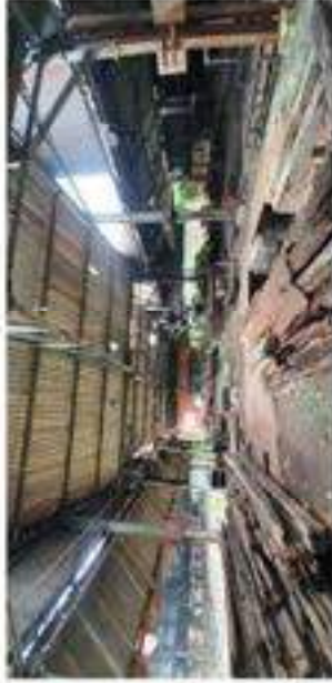
Condition of iron columns in low mill structure
