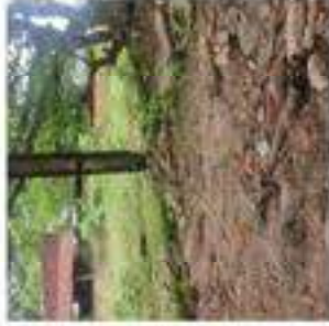
Corroded iron columns
