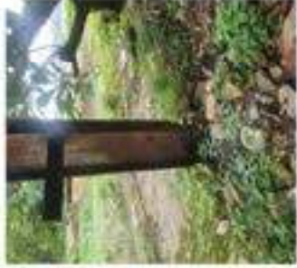
Highly distressed condition of columns
