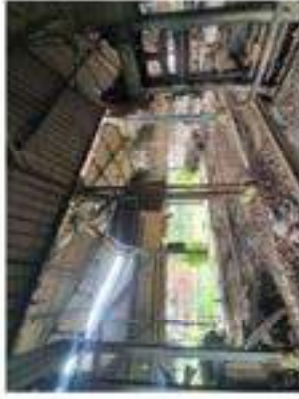
Corroded iron columns
