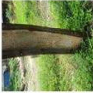
Prominent geometric deformation of iron column
