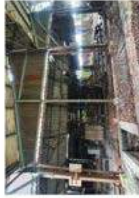
Floor condition of iron truss in low mill
