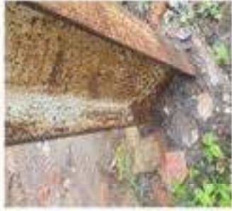
Highly distressed condition of iron
