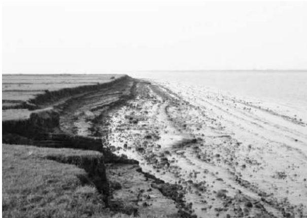
Erosion at Shalukkhali
